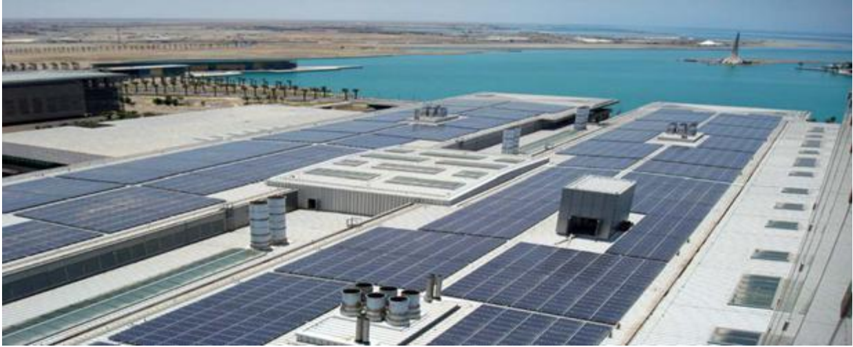
2MW rooftop solar park, KAUST University, Saudi Arabia
